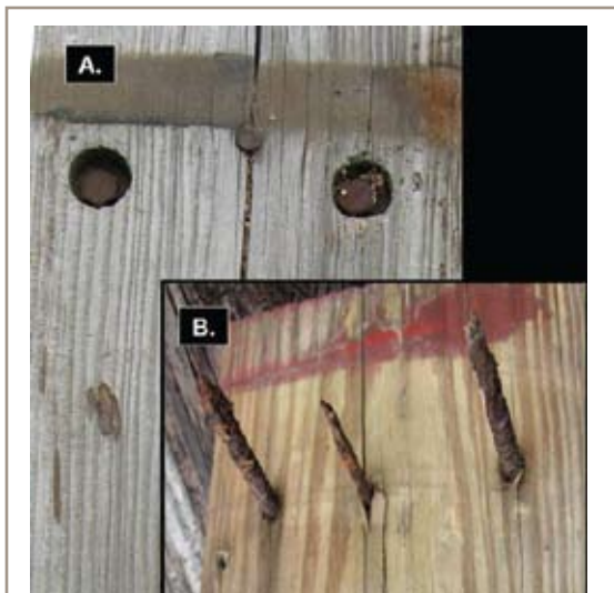
Figure 3. (A.) shows a top view of 3 ½ inch treated lag screws and a nail inside the decking, (B.) is the bottom view of the same board withdrawn from its support on a 28 year old deck. In (B.) the corrosion of the lag screws (no threads) and nail have allowed the decking to move freely on its supports which was common to the majority of the boards on the deck. Notice the splitting near the end grain where moisture is absorbed by wood and where fasteners are used for connection to the deck framing.
