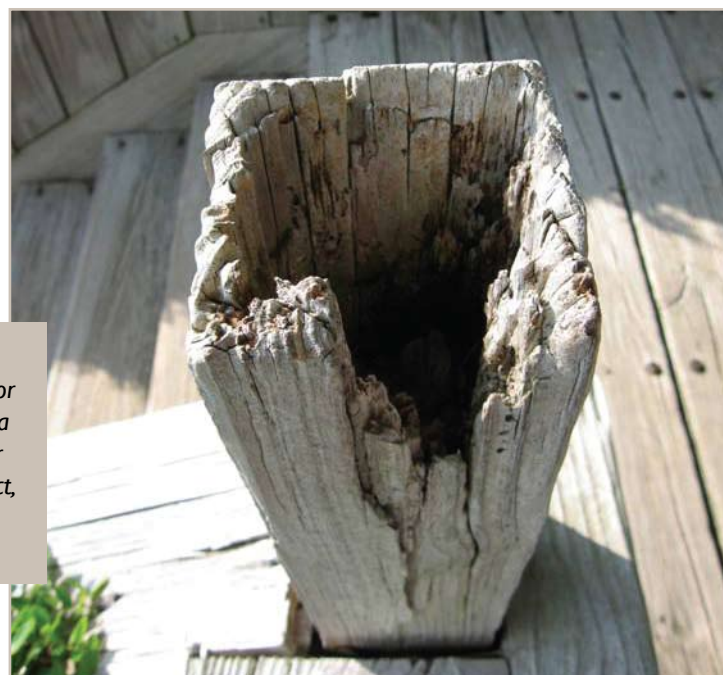
Figure 5. A cap (circle) or railing board (arrow) should cover exposed end-grain of wood, after treatment with a water-repellent preservative, to deter moisture from pooling on the end-grain of the wood.
