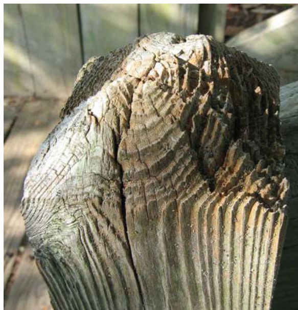
Figure 10. In contrast to the post shown in Figure 6, this post on the same deck was cut at the top to shed water and experienced much less decay.
